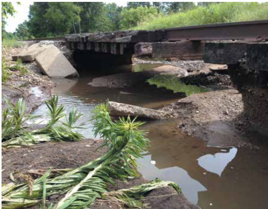
Erosion and flooding can cause damage missed by aerial patrols 1,700 feet or more in the air. Comprehensive ground right-of-way patrols by trained technicians can spot such damage before a rupture occurs. Source: Atlas Field Services LLC
