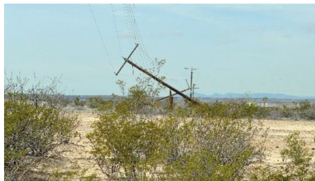
Failed electrical infrastructure, like this one in the Permian Basin, often goes unnoticed until there is a significant event or disruption to the system. (Source: Burns & McDonnell)
