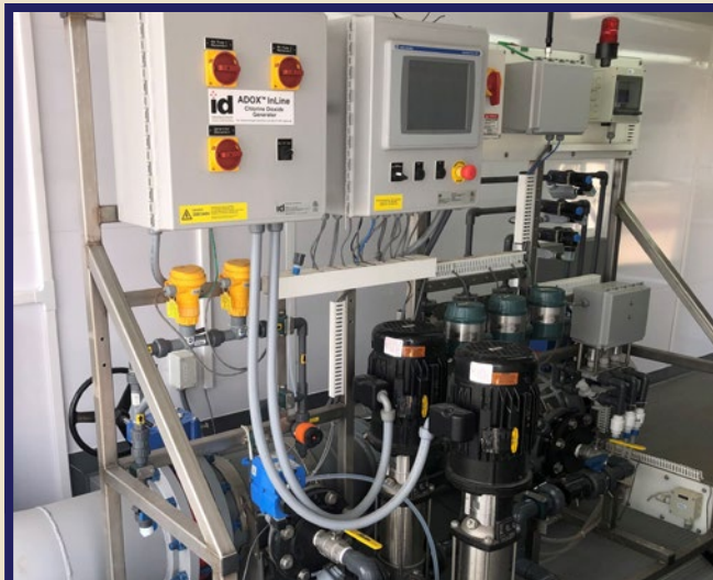
The 12-inch inline \text{ClO}_2 generation technology is shown being deployed for frac on the fly. (Source: International Dioxide)
