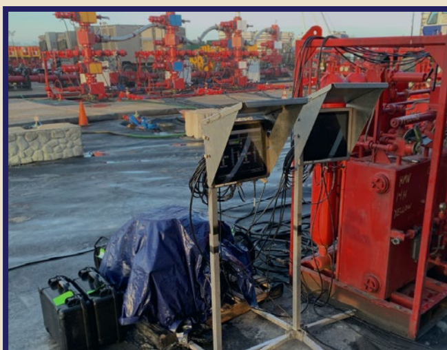
Using sensors, SmartPAD tracks operations directly at the wellhead and connects all onsite service companies to a trusted source of formatted and time-stamped operational data. (Source: Cold Bore Technology)
