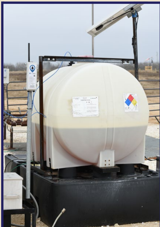
WellAware On Demand Chemical is installed on a tank in a field to automate chemical injection. (Source: WellAware)
